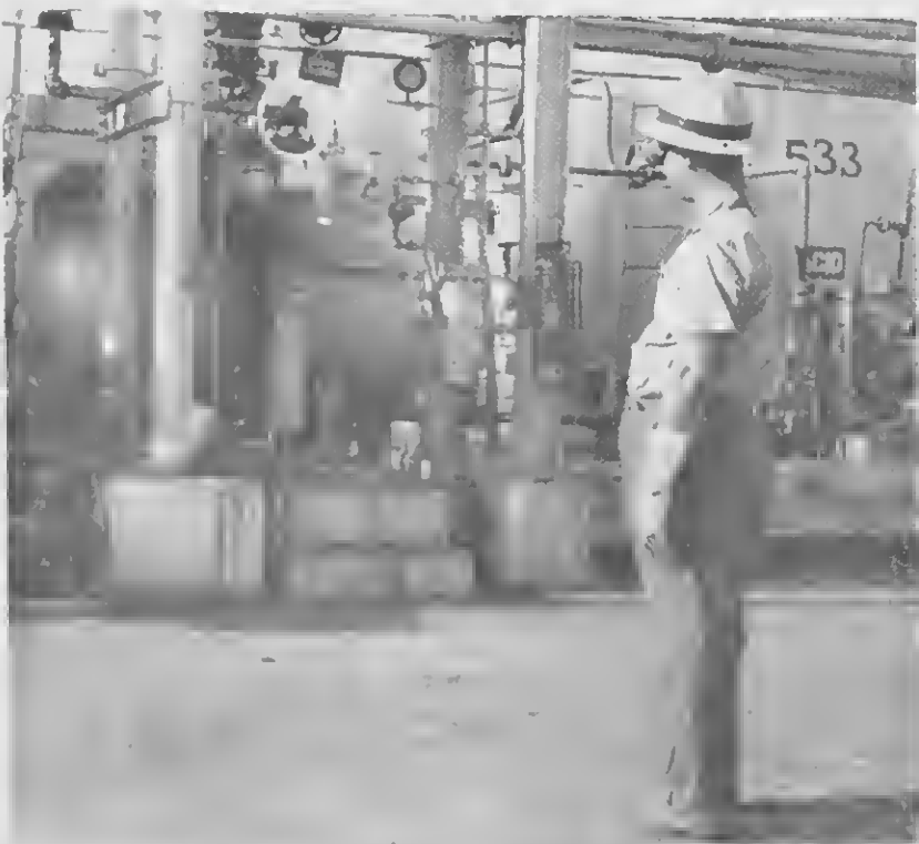
THE SCENE: The infamous spray broke loose from a connection in the piping shown by the arrow and circle. Mr. Montnor's approximate position is shown by a fellow worker. Although some 20 to 25 feet away from the break, he was hit on the upper left side of his body by the stream. The acid splashed over his body and on his face, but, thanks to his safety goggles, his eyes were completely protected from injury.
